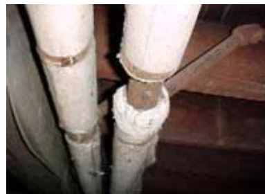
Asbestos-Containing Pipe Insulation
