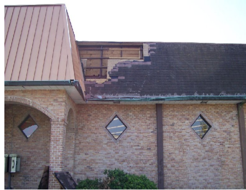
Hurricane Damage - Exterior
